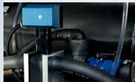
Servo-controlled three-way hydraulic valve.
